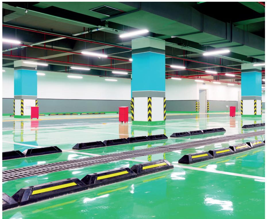
Indoor Parking Lighting
